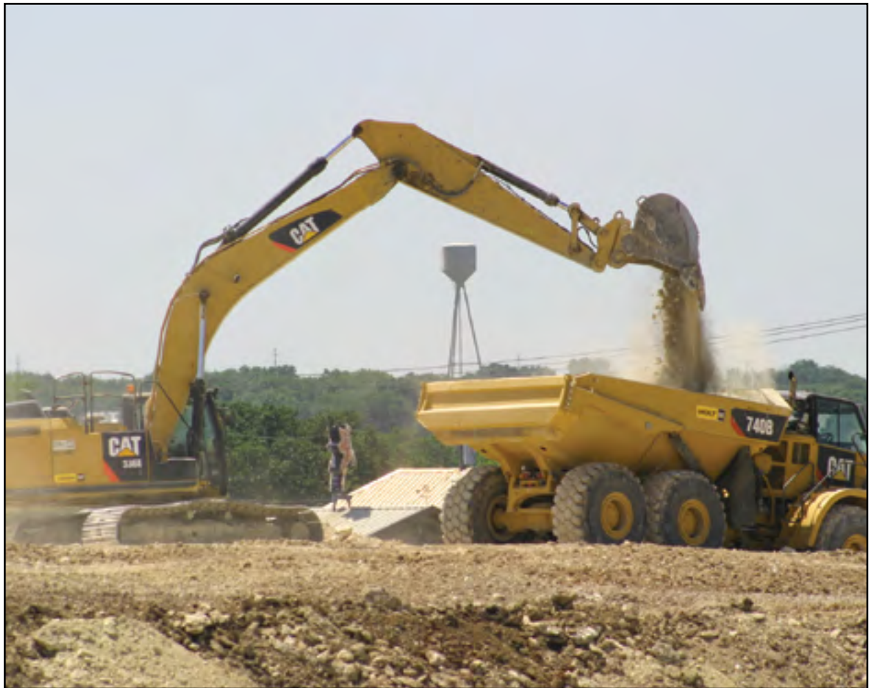
James Construction is expected to begin working on the Salado Plaza underpass at I-35 within the next few weeks and have it completed by the end of the year. (PHOTO BY ROYCE WIGGIN)
