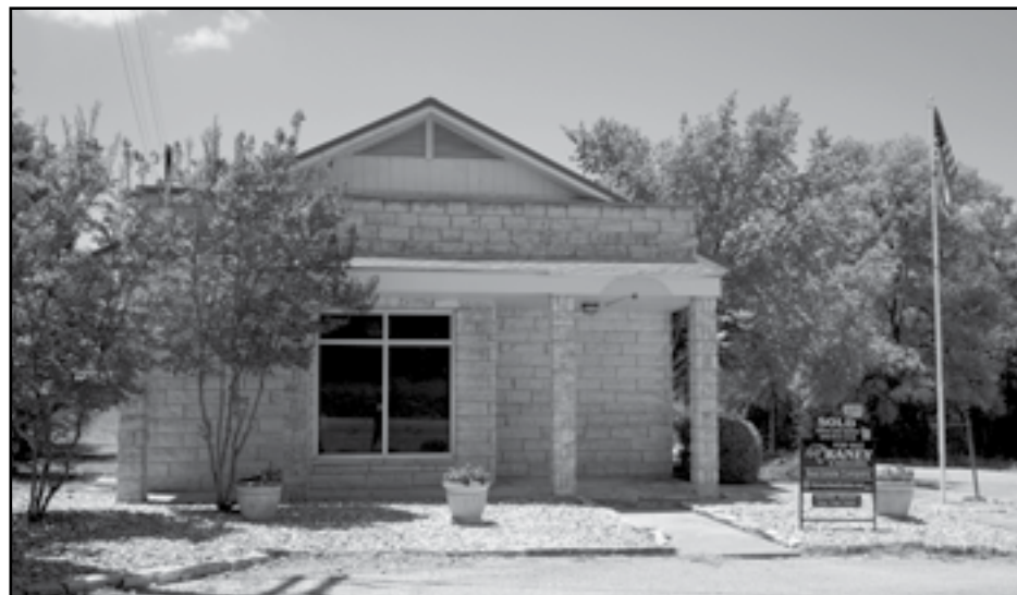
Renovation has begun on the building which was once home to the Salado Post Office. Most recently it housed Ronnie Wells Gallery. PHOTO BY LATRAYA LUKE
