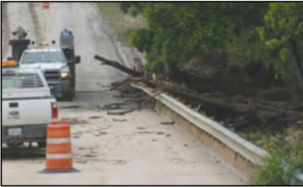
The flooding of Salado Creek on May 25 caused damage to the southbound access road bridge, requiring its closing. More than six months later, the access road is still closed. (PHOTO BY ROYCE WIGGIN)
