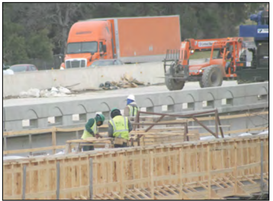
A Feb. 1 deadline looms for the opening of the southbound access road south of Thomas Arnold to FM 2268 Holland Road overpass. The road has been closed since May 2015. If PCS/James Construction work crews meet the deadline, the access road on the east side of I-35 south of Thomas Arnold will become one-way, northbound. The next critical deadline is March 11 to open Salado Plaza east-west traffic on the new temporary connection. (PHOTO BY ROYCE WIGGIN)
