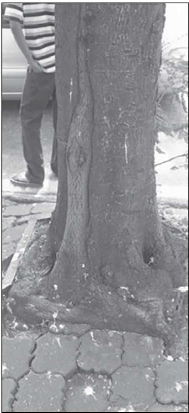
Tree roots can damage sidewalks, parking areas and even the foundations of buildings. (COURTESY IMAGE: WILLIAM FOUNTAIN, UNIVERSITY OF KENTUCKY, BUGWOOD.ORG)
