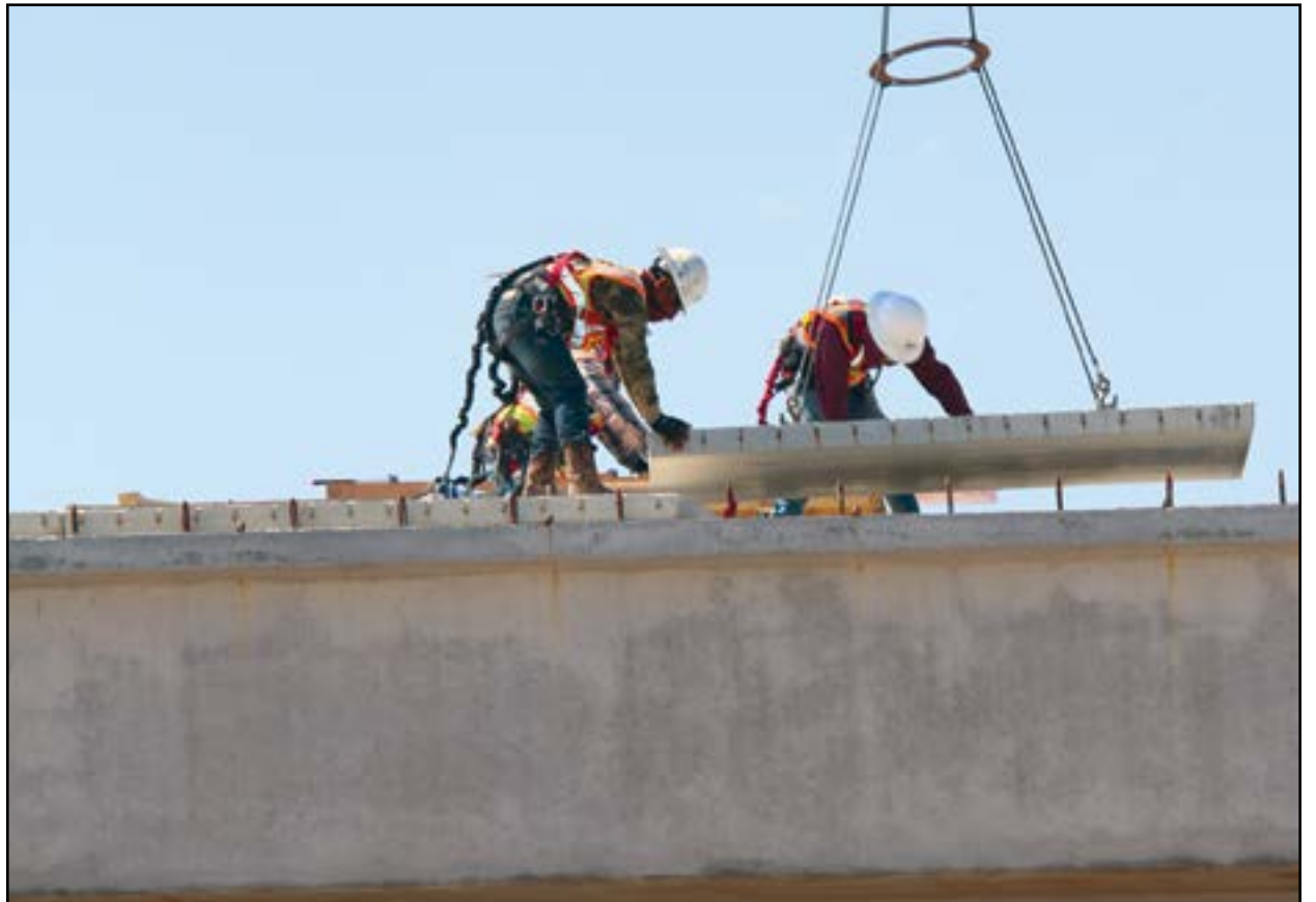
James Construction crews work on the Salado Plaza overpass of I-35. James Construction missed its milestones of March 11 for the completion of the Salado Plaza east-west temporary lanes. All traffic lanes were open, as well as all exits and access road lanes, as of Thanksgiving. Minor work remains to complete the expansion project, which is now a year-and-a-half late. (PHOTO BY ROYCE WIGGIN)
