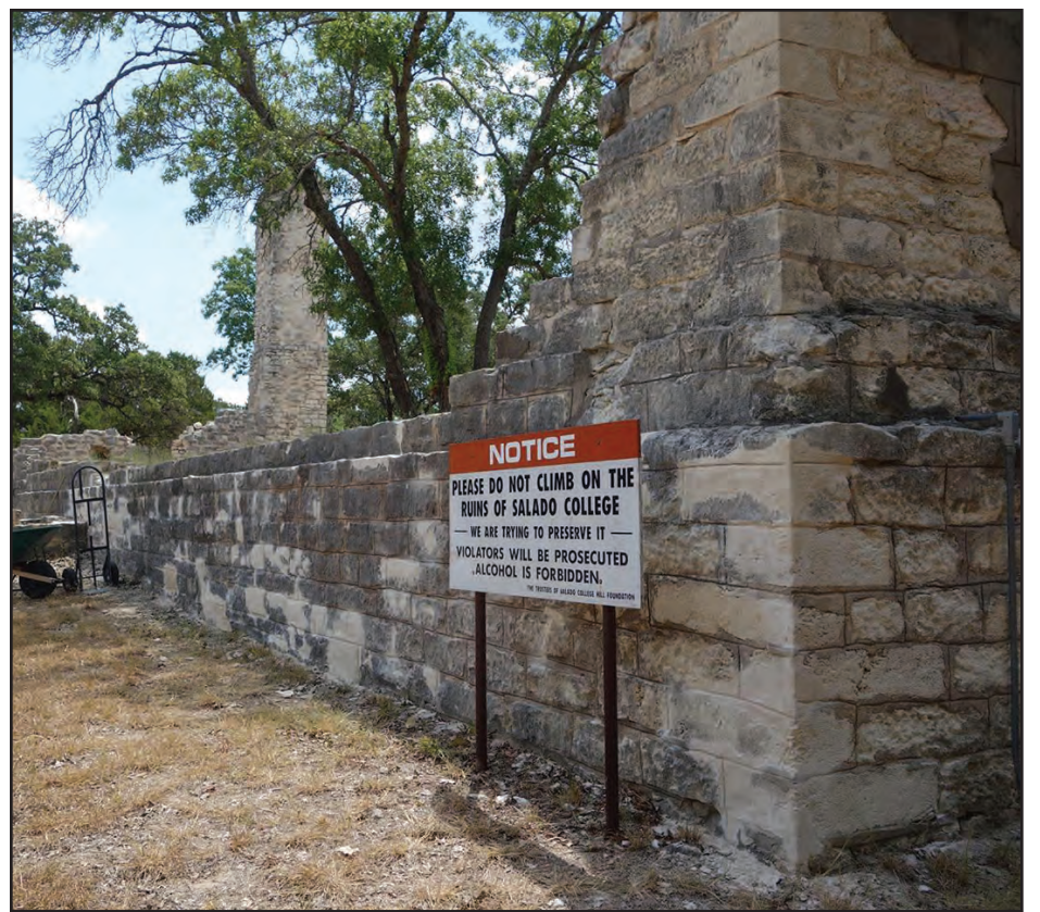
Light spots in the stone show where mortar work has recently been completed on the Salado College ruins.
