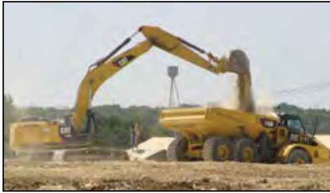
The I-35 construction project through Salado has gone on two years beyond the contract end date of Spring 2015. (FILE PHOTO BY ROYCE WIGGIN)
