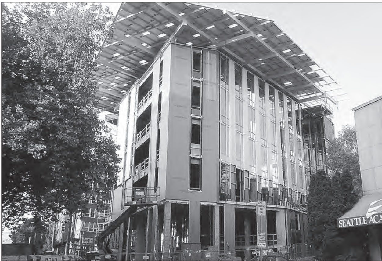
PHOTO BY JOE WOLF, COURTESY FLICKR So far, 15 different projects, from New York State to Hawaii, have been certified as "Living Buildings." The likely 16th is Seattle's Bullitt Center (pictured here in progress), a six-story solar-powered "net zero" building designed to make extensive reuse of rainwater and day lighting and which features many other green amenities.
