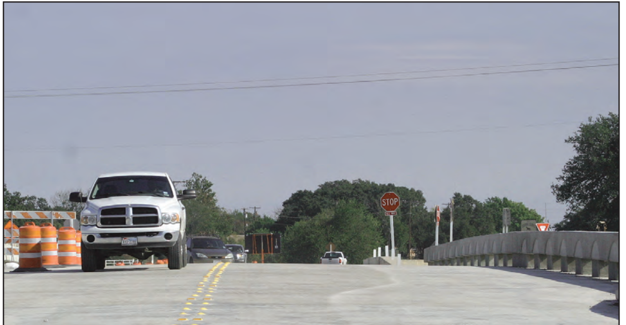
The FM 2268 new bridge structure opened Nov. 12 after the old bridge was demolished overnight Nov. 11 requiring a mainlane closure. James Construction has set the date for the demolition of the Thomas Arnold bridge as Dec. 16. (PHOTO BY ROYCE WIGGIN)
