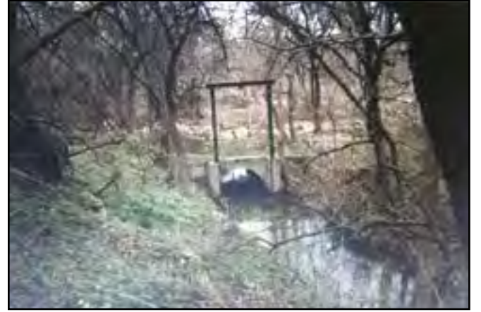
Ike Jones Mill sluice gate located near Amity Road East. The opening of the sluice gate started the water on its way to the mill. (PHOTOGRAPH COURTESY OF DR. DAVID J. MIKULENCAK)
