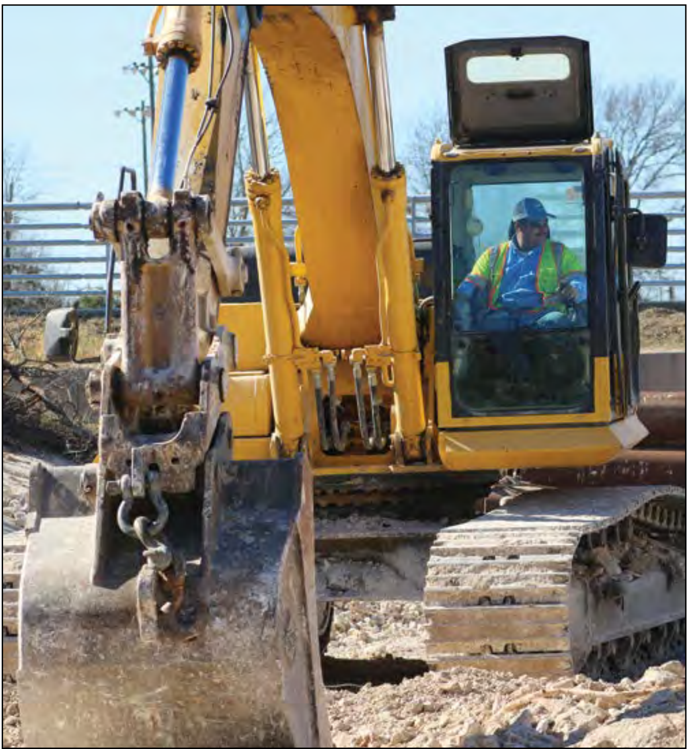
Heavy work has begun on the Salado Sewer project. A work crew is shown above digging in the seasonal creek bed between Stagecoach Rd. and Church St. The collection pipe connecting the east and west side of the sewer system will go under I-35 and the access roads at this location. (PHOTO BY ROYCE WIGGIN)
