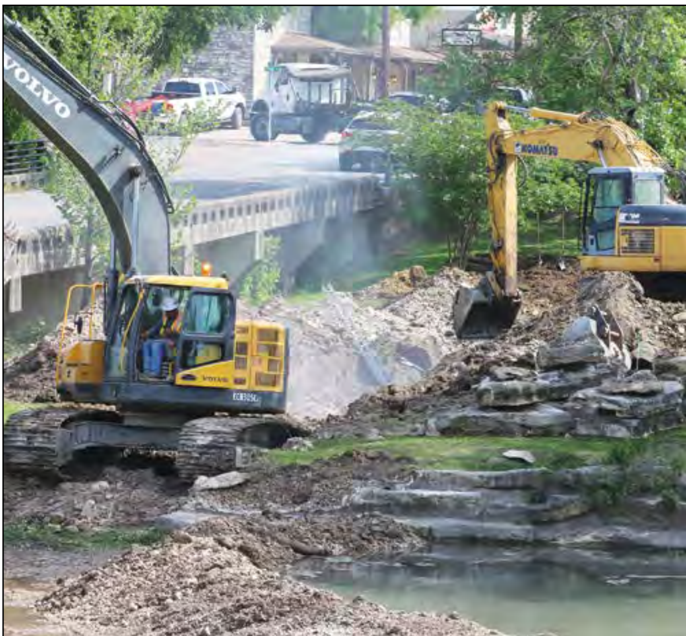
McLean Construction crews laid sewer pipes across Salado Creek last week, damming half of the creek at a time in order to dig open trench for the pipeline to serve Main Street. The work began early last week and took just a week to complete trenching, laying pipe and recovering. Crews are now trenching and laying sewer pipe along Main Street right of way. (PHOTO BY ROYCE WIGGIN)
