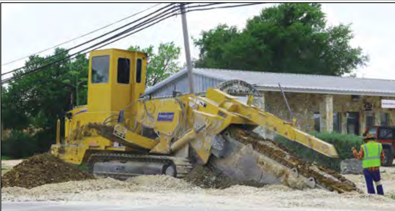
McLean Construction has completed work on the sewer collection system on Royal Street, south Main across Salado Creek, and Church Street. Crews have worked their way up Main Street to Blacksmith and are expected to finish the rest of the Main Street collection system before starting on West Village Road and the collection lines on the west side of the interstate. Village administrator Don Ferguson is meeting with owners of properties on the west side of the interstate who have expressed interest in tying in to the sewer system. The treatment plant is on schedule for completion by mid-January, Ferguson told Aldermen June 21. The collection system, which has hit delays because of rock formations, utility conflicts and delivery of a lift station, is expected to be complete by mid-March 2019. No reports from the Village on when Sanctuary development will begin. The Village has wastewater services agreements, economic development agreements and tax abatement agreements with Sanctuary. (PHOTO BY ROYCE WIGGIN)
