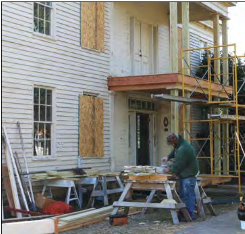
Work began in 2017 on the restoring the exterior of the Halley House, owned by Kathy Michael. (PHOTO BY TIM FLEISCHER)
