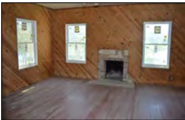
This photograph shows the renovation of the front parlor. The walls have been restored to their original ship-lap boards and new windows have been installed. (PHOTO BY MAURICE CARSON, MAY 6, 2018.)
