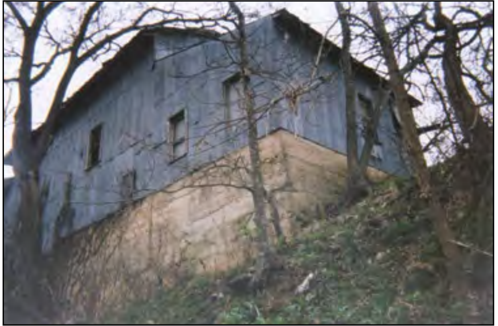
This 1995 photograph shows the creek-side of the abandoned Ike Jones Mill. The mill was in operation from 1880 to 1917. (Photograph courtesy of Dr. David J. Mikulencak.)
