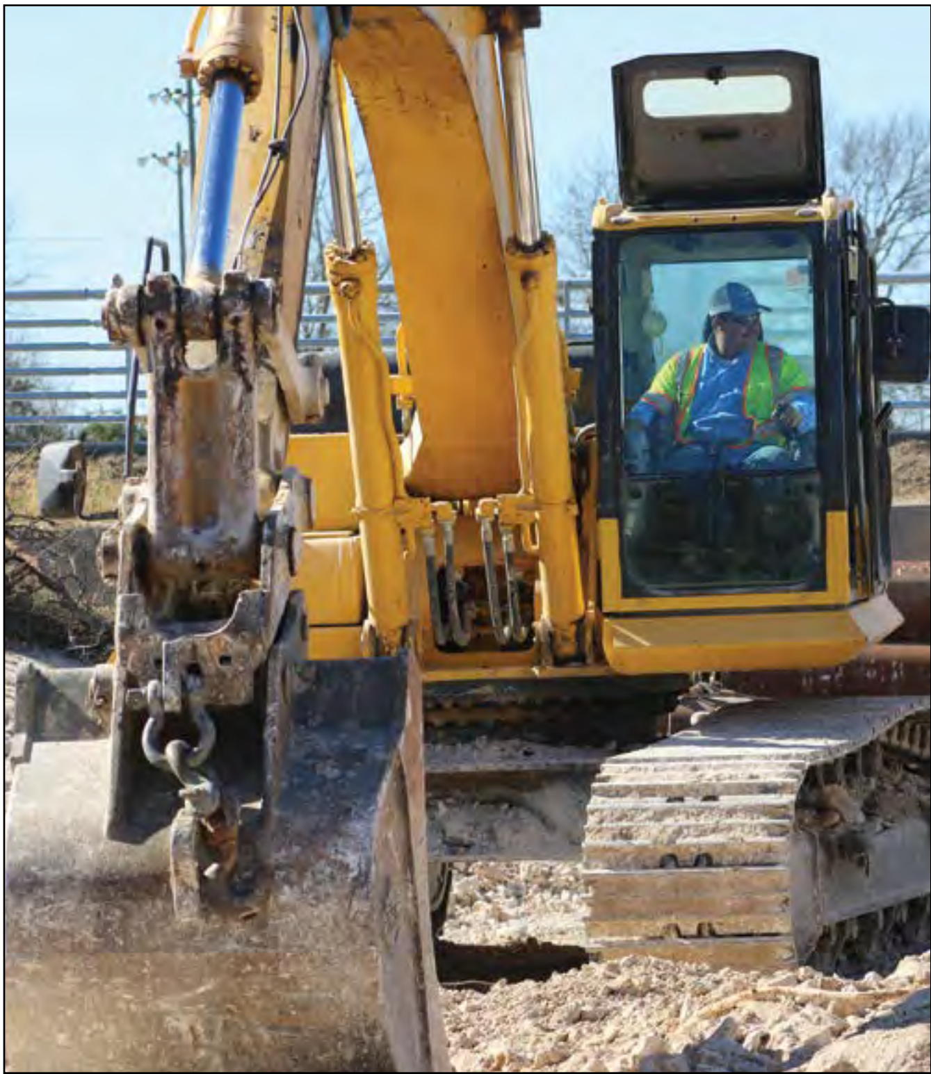
Heavy work began in late January on the Salado Sewer project. A work crew is shown above digging in the seasonal creek bed between Stagecoach Rd. and Church St. The collection pipe connecting the east and west side of the sewer system goes under I-35 and the access roads at this location. The work continued throughout the year and the collection system is now 99 percent complete, according to Village Administrator Don Ferguson. End users will begin tying in to the system in early 2019. (PHOTO BY ROYCE WIGGIN)
