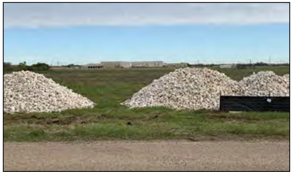
This is a picture of the future site of the new middle school and the new baseball and softball complex on Williams Road. Our current high school is in the background.
