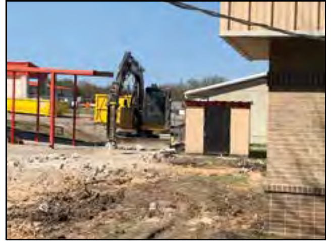
This is a picture of the construction at the elementary school on Thomas Arnold Road.
