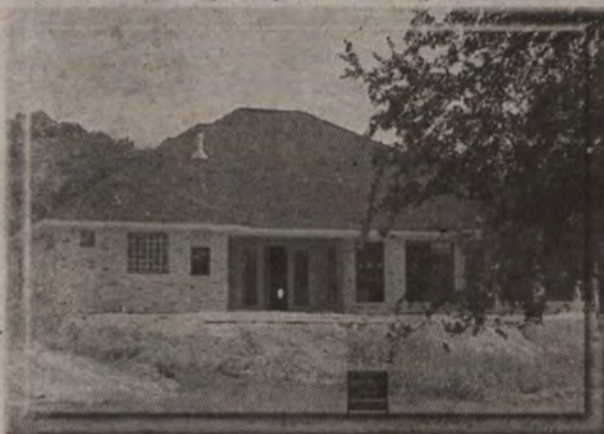
New home under construction on the golf course overlooking Salado Creek. Absolutely beautiful view. Ten to fourteen foot ceilings thruout the home. Priced at $310,000.
