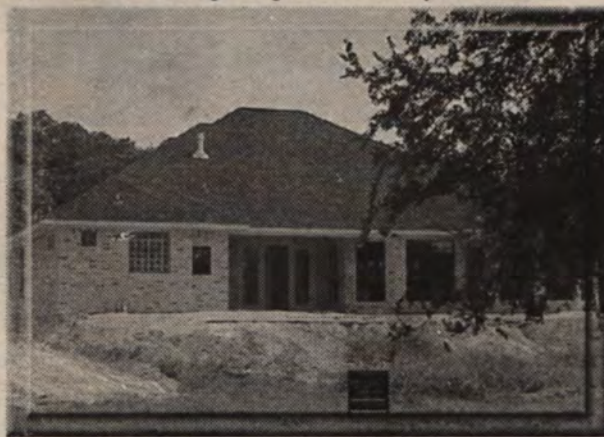
New home under construction on the golf course overlooking Salado Creek. Absolutely beautiful view. Ten to fourteen foot ceilings thruout the home. Priced at $310,000.
