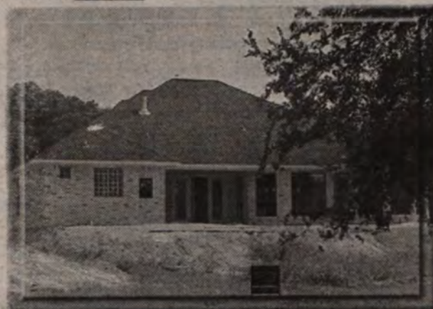
New home under construction on the golf course overlooking Salado Creek. Absolutely beautiful view. Ten to fourteen foot ceilings throught the home. Priced at $310,000.
