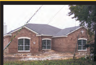
$174,800: Unique kitchen design is roomy with large pantry and island. Master BR with window seat and TV niche. Formal dining plus breakfast room. Split bedrooms.
