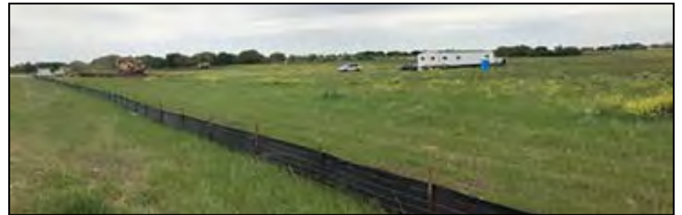
This is the site of our new middle school and baseball/softball complex. The job site trailer is set up. Earth work equipment is on site and they have begun moving dirt.
