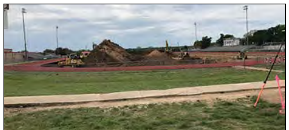
This is the football/soccer/track stadium renovation. They are working on the foundation prior to installing artificial turf.
