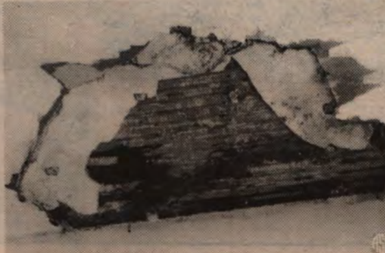
Often, homeowners don't realize pests are damaging their homes until it is too late. Much of the damage caused by termites can only be found by looking behind the walls.
