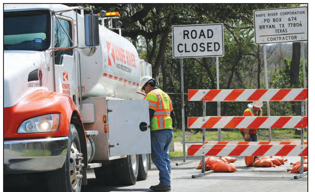
The bridge of Salado Creek for East Amity was closed from early March until the fall as the low water bridge was replaced. Knife River Corporation-South, of Bryan, undertook bridge replacement project at a cost of $1.2 million. (PHOTO BY ROYCE WIGGIN)
