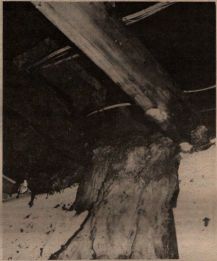
Burned insulation in the attic of the Stagecoach Inn hotel is shown above. The hotel caught fire Oct. 9 with damage to 15 rooms. (photo by John Eubanks)
