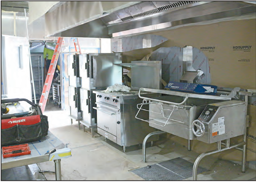
State of the art equipment in the Cafeteria kitchen at Salado Middle School.
