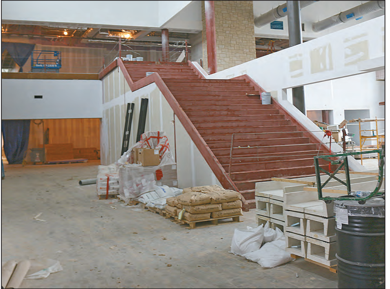
A stairway that looks into the two-story library is a central design piece in Salado Middle School.
