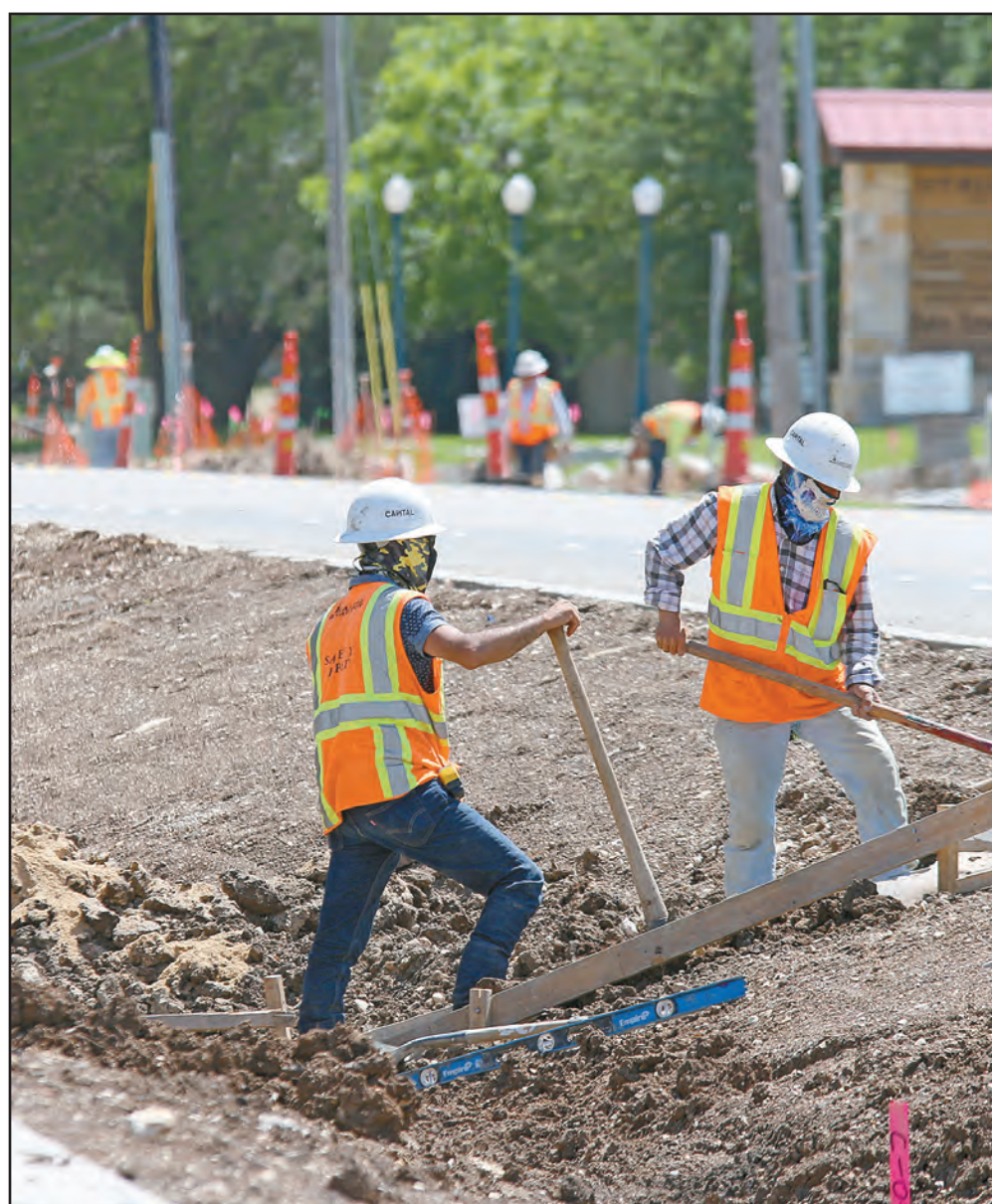
Austin Excavation workers work on the swale between the road and the sidewalks. The Main Street project is on schedule for completion this summer. (PHOTO BY ROYCE WIGGIN)
