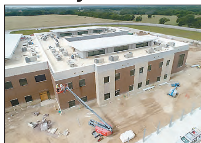
(COURTESY SALADO ISD) Aerial view of brick and stone going up at Salado Middle School. The contractor is on pace for substantial completion to open for the 2020-2021 school year.
