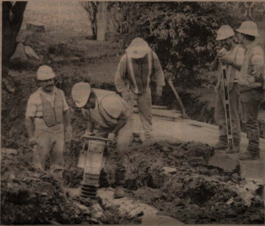
Work continues on the widening of the Main Street walkway bridge, which is expected to be completed later this year. (Photo by John Eubanks)
