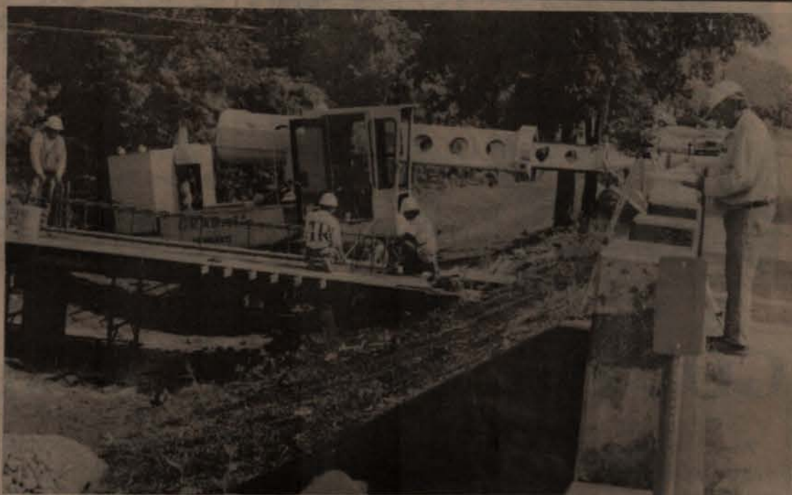
Work continues on the bridge and walkway project. (photo by John Eubanks)
