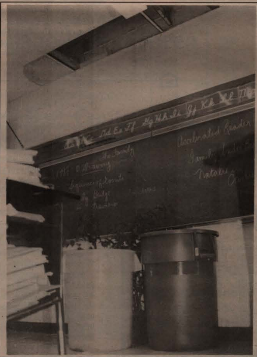
Unfortunately, the sight of trash cans throughout the school (to catch leaks caused by deteriorating roofs) is a regular sight after most rains on Salado schools.
