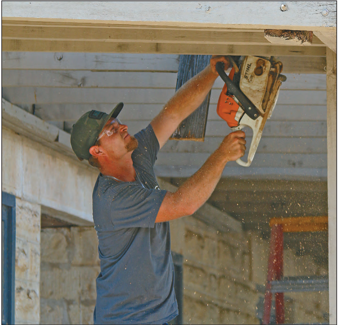
Sandor Construction crew began the demolition of the balcony at Salado Museum on Aug. 6. The old balcony is being replaced as a major project of the Salado Museum. (PHOTO BY ROYCE WIGGIN)
