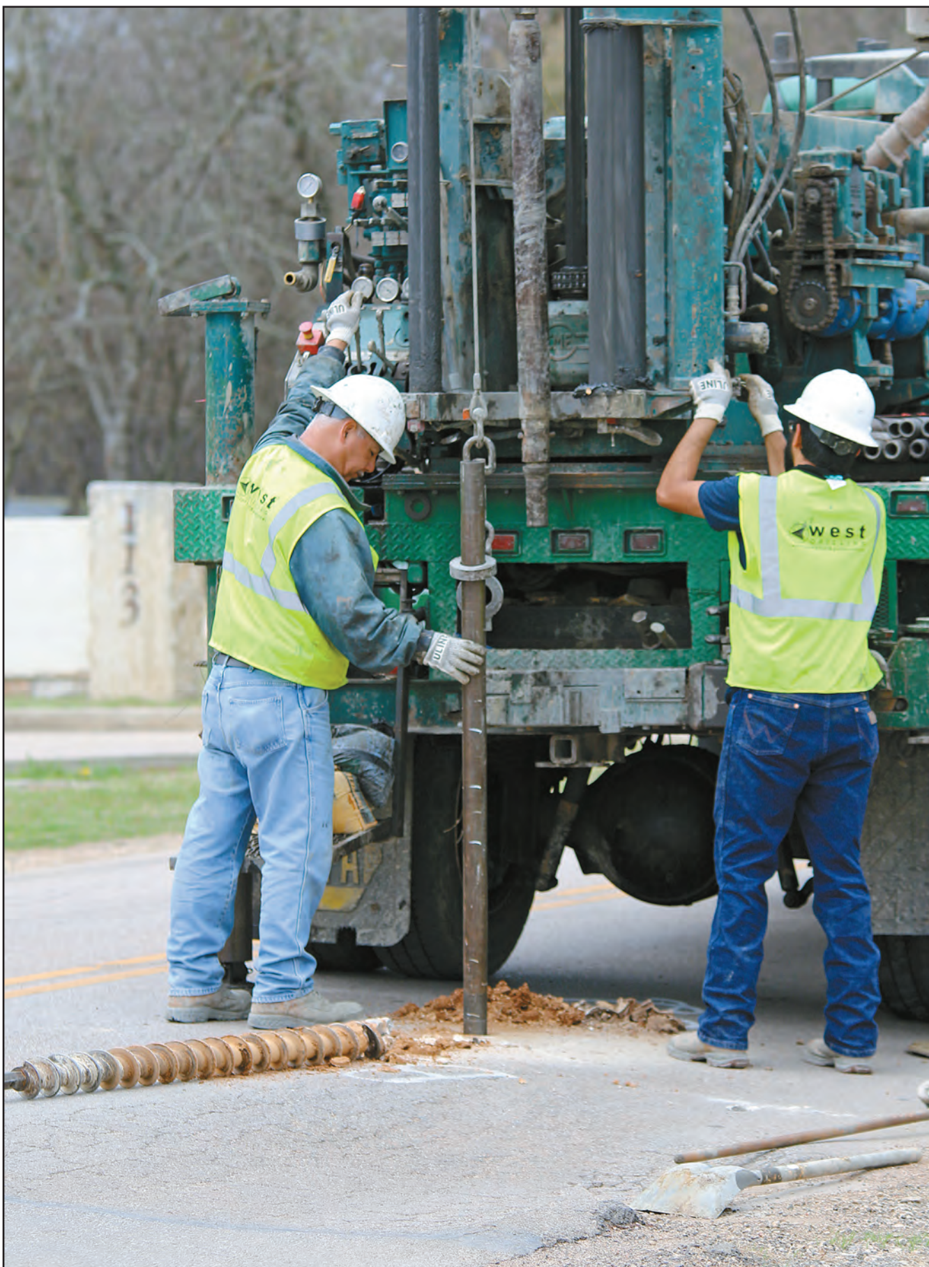
Work crews began repairing pot holes on Salado Plaza Dr. this week. As the weather grows warmer, look for state, county and local crews to begin work on the area streets and roads. (PHOTO BY ROYCE WIGGIN)
