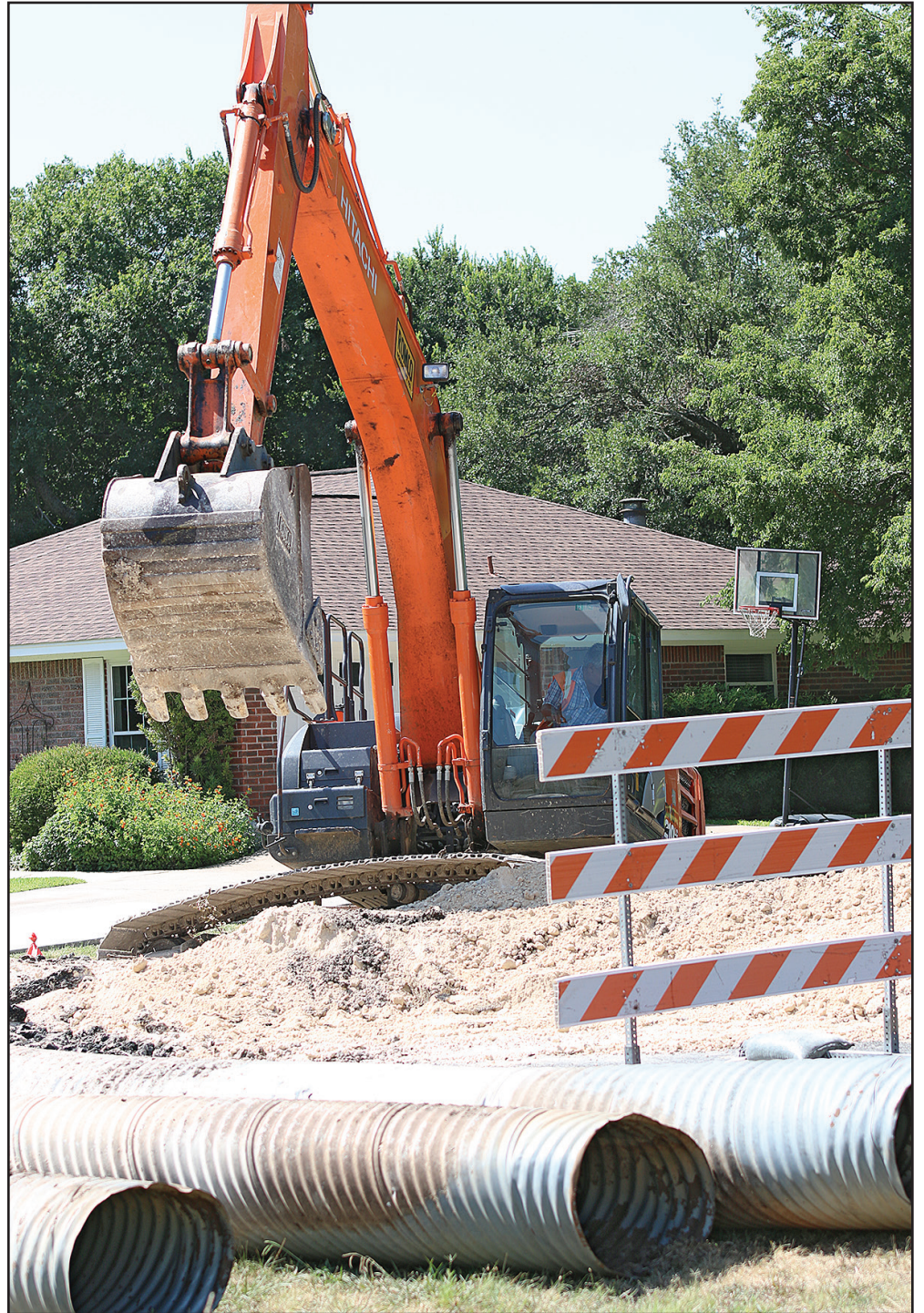
Work began last week to replace the culverts on Mill Creek Dr. to mitigate flooding concerns on the main road out of Mill Creek. The road will be closed for the duration of the project, which is anticipated to take six weeks. (PHOTO BY ROYCE WIGGIN)
