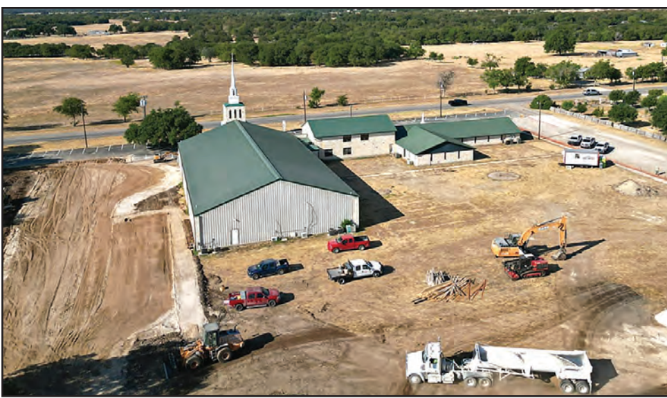
Work has begun on a $4 million capital improvement project at Grace Church of Salado. (COURTESY PHOTO)
