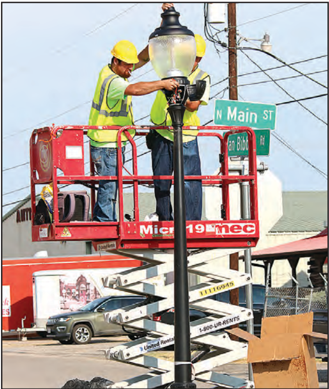
Crews began replacing the streetlights on Main St. earlier this week. (PHOTO BY ROYCE WIGGIN)
