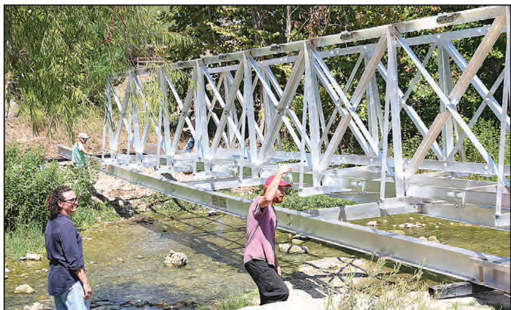
(PHOTO BY ROYCE WIGGIN) KD Hill watches as Barrow Brewing Co. workers install a walking bridge to span Salado Creek. The bridge will alleviate pedestrian traffic jams during peak weekends as well as connecting the southside of downtown Salado to parking in Pace Park.
