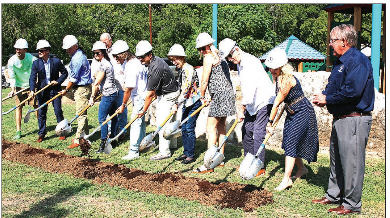
The Village of Salado broke ground on the construction of an All Abilities Playground at Pace Park on Oct. 2, with representatives from the board of aldermen, Sirenafest, Variety Peaceable Kingdom Retreat for Children, Mustang Springs at Salado, the Morris Foster Foundation, and Legacy Salado, Inc. and the Village Parks advisory board. Construction is expected to be completed by March 2024. Shown above, from left are alderman Jason Howard, Jonathan Briscoe, board member of Variety Texas Peaceable Kingdom Retreat for Children, alderman Bert Henry, Theresa Howard with Legacy Salado, Jim Kerby, principal of Kerby Investments and Mustang Springs at Salado, which donated $360,000 to the effort, alderman Jasen Graham, Lyn Haney with the Morris Foster Foundation, Amber Preston Dankert with Legacy Salado and member of the Parks advisory board, alderman Paul Cox, Tiffany Schreiner, founder of Sirenafest and mayor Michael Coggin. (PHOTO BY MARILYN FLEISCHER)
