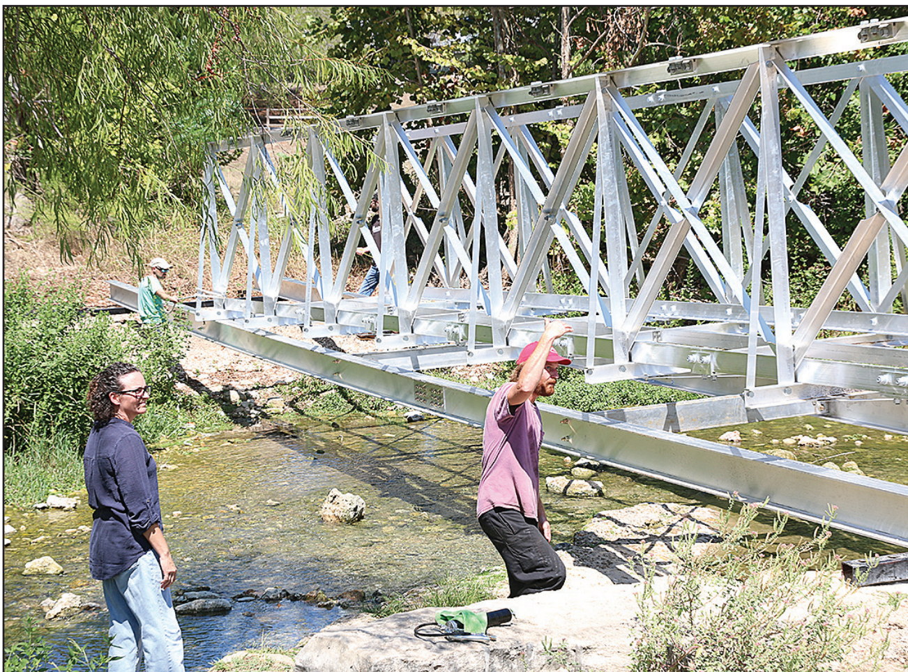
KD Hill watches as Barrow Brewing Co. workers install a walking bridge to span Salado Creek. The bridge will alleviate pedestrian traffic jams during peak weekends as well as connecting the southside of downtown Salado to parking in Pace Park. (PHOTO BY ROYCE WIGGIN)
