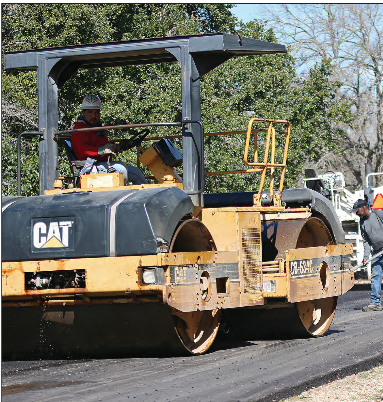
Road crews began work last week on resurfacing Center Circle. Crews have also begun work on the drainage project at Chishom Trail and Stagecoach Circle. (PHOTO BY ROYCE WIGGIN)
