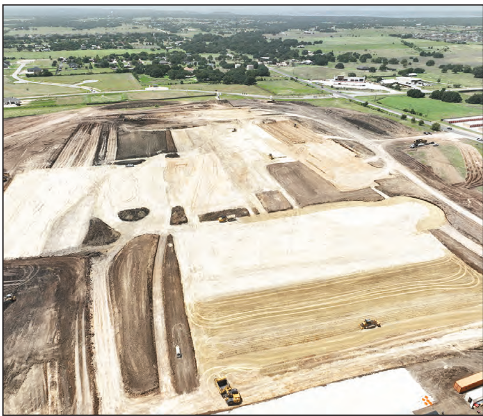
COURTESY PHOTO Site grading begins to show the footprint of the new Salado High School
